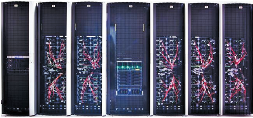
Figure 2. The KID system as installed in Keeneland's data center. The compact 201 teraflops/s system requires only seven racks and 90 square feet of floor space.
